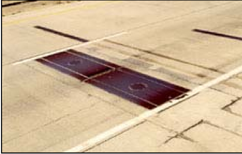
Figure 2-6. Typical Installed Weigh-In-Motion Pad.
