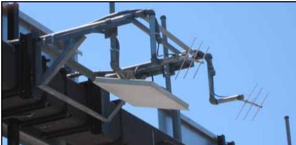
Figure 2-2. Transponder Reader Antenna (flat panel) and E-Seal Reader Antennas (3-prongs each) Installed at the Northbound Crossing Overhang.
