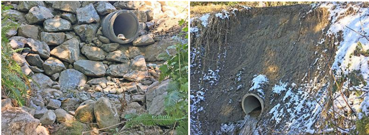
Above left: Photo shows scale of fish barrier at the outlet of the culvert. Above right: Photo shows prior damage when the downstream end of the culvert failed and temporary repairs were made to prevent loss of the roadway.
