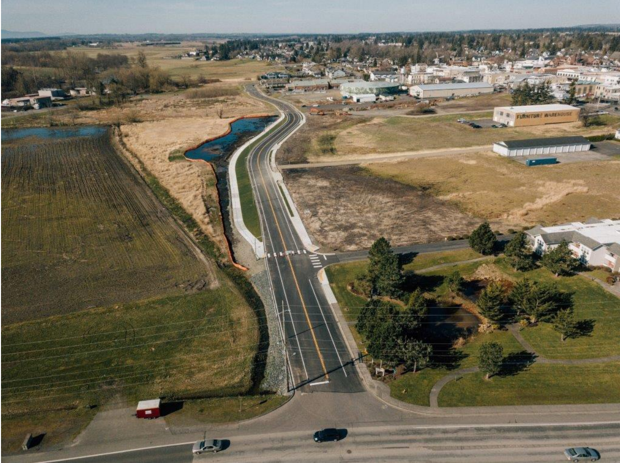
City of Lynden recently finished the new roadway construction of Riverview Rd that connects the S 6th St to Hannegan Rd.
