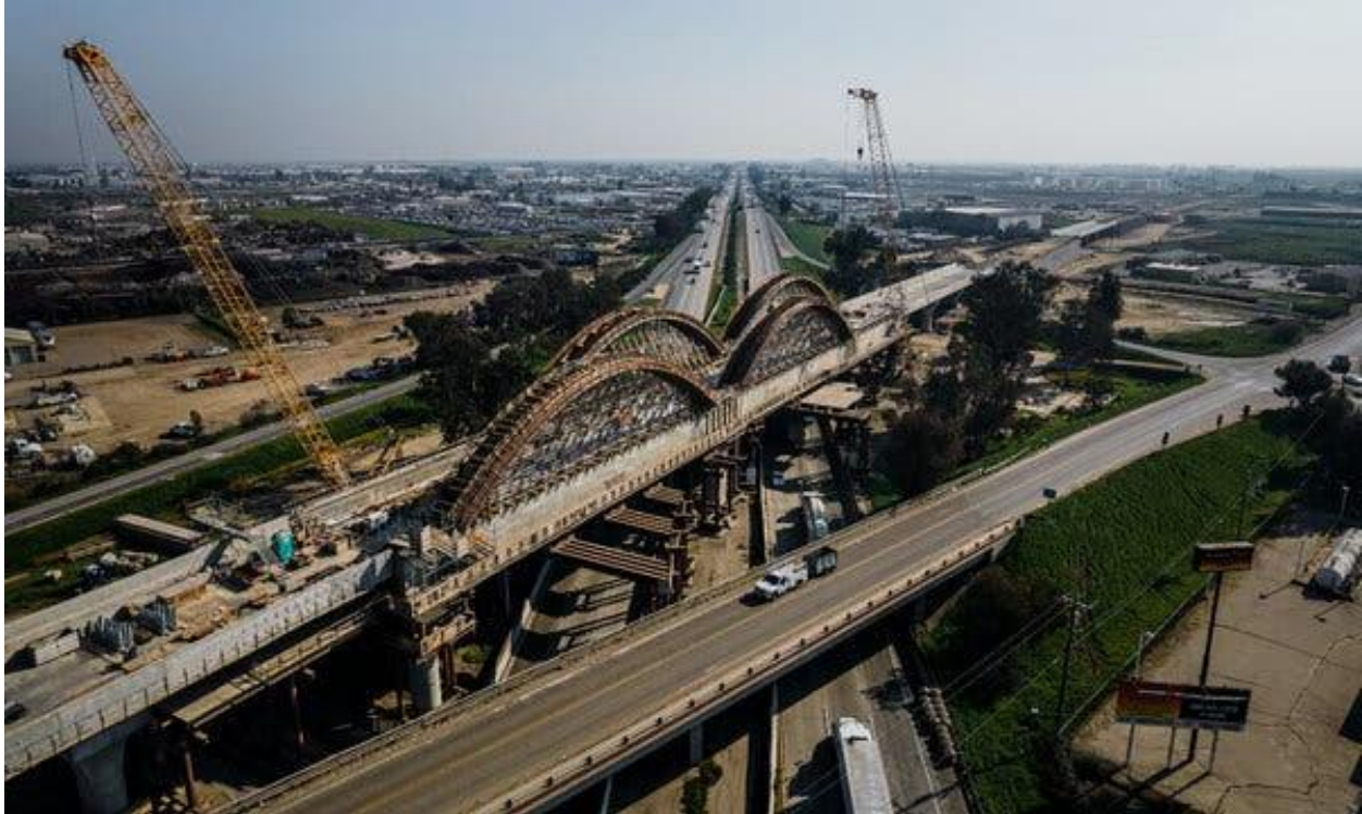
A number of viaducts for the high-speed rail system are in various stages of construction in the Central Valley. Ryan Christopher Jones for The New York Times
